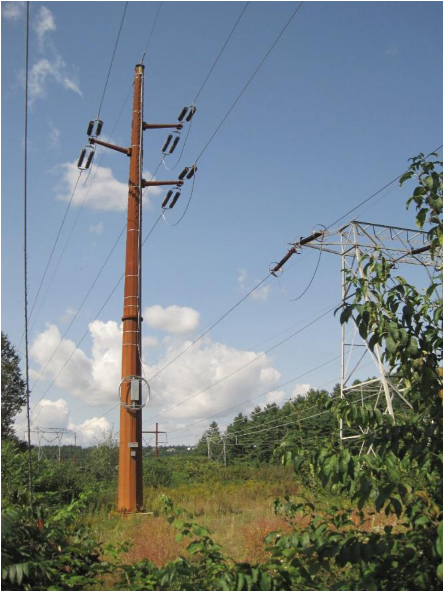
Transmission Pole 52 MVRP
